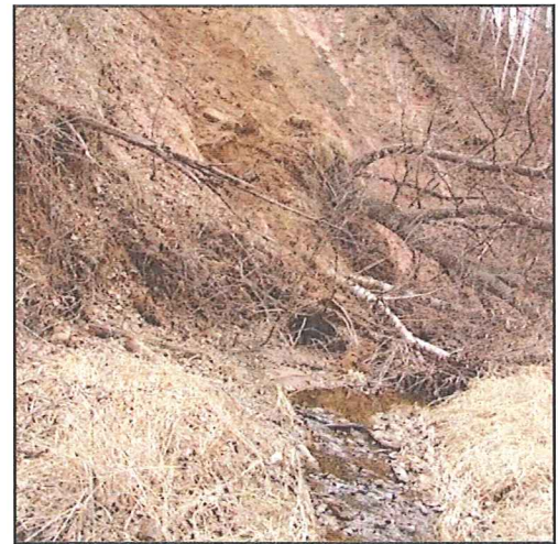
Eroding Bank Gully of County Ditch 9
