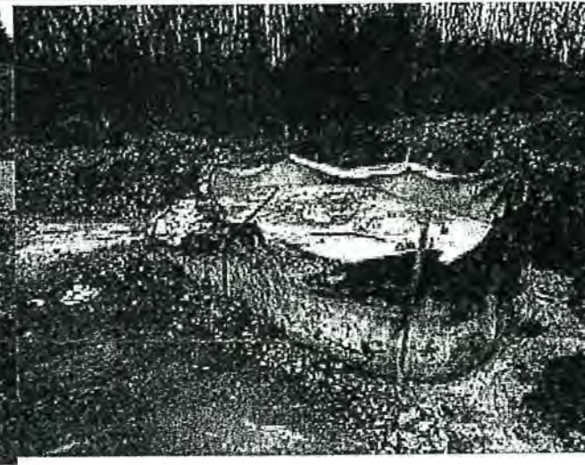
Concrete washout tote
