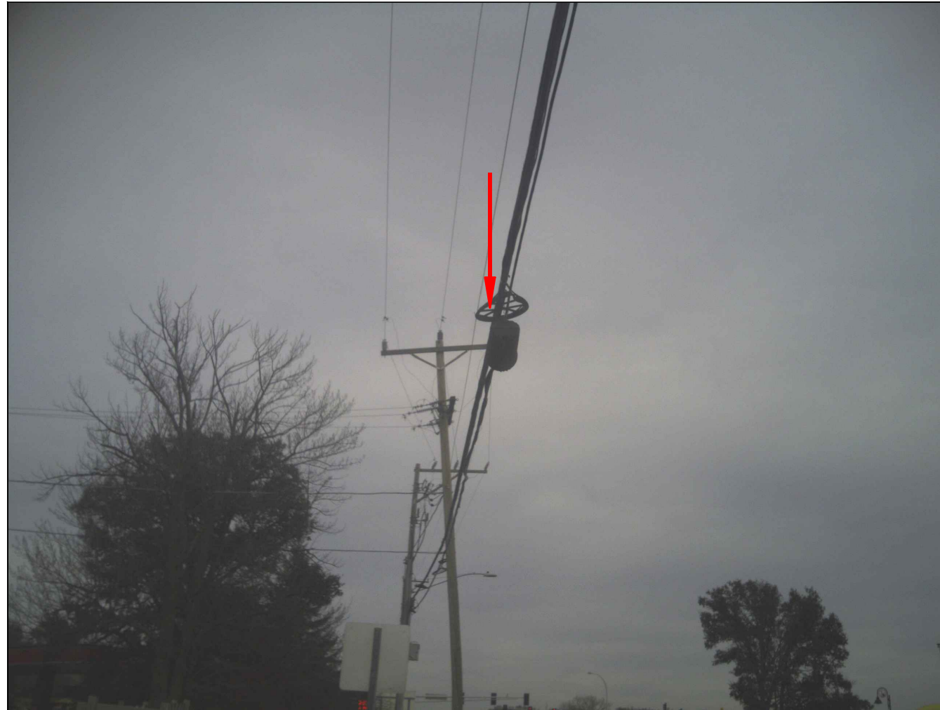
Existing Splice Case
