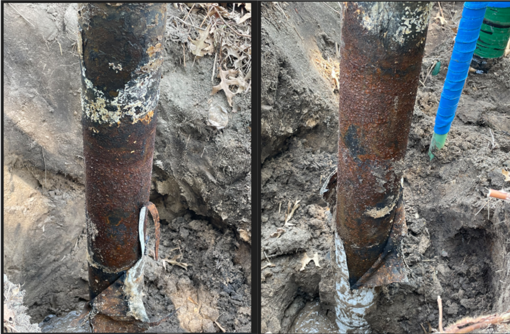
Images from Xcel CP tech regarding general corrosion on hair pin to reg. Coating determined to be field applied cold wrap. No info on condition of pipe after transition to factory applied coating.
