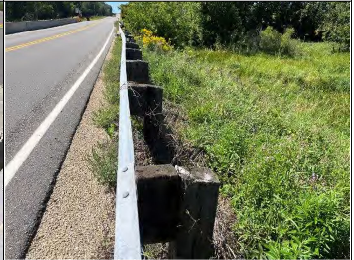
Photo 4 – View of creosote-treated guardrail posts and spacers along the north guardrail.
