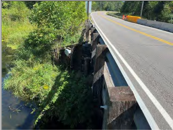
Photo 5 – View of creosote-treated guardrail posts and wing wall along the north guardrail.
