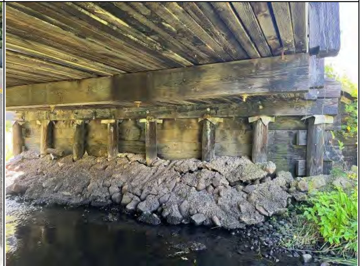
Photo 6 – View of treated timber construction below Bridge 02502 including abutment, pilings, and slab.
