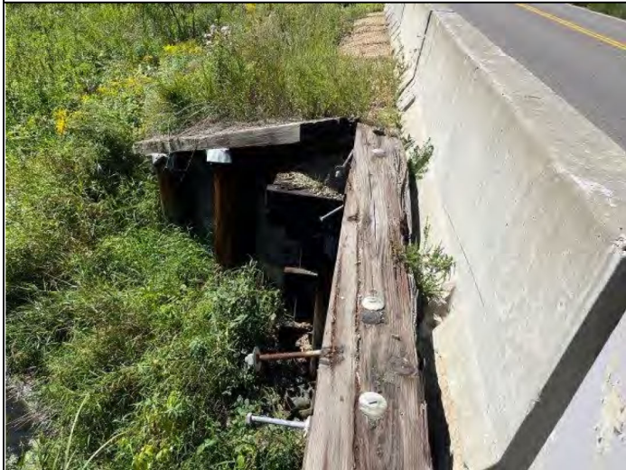
Photo 3 – View of creosote-treated timber curb and wing wall at the south and southwest portions of the bridge.
